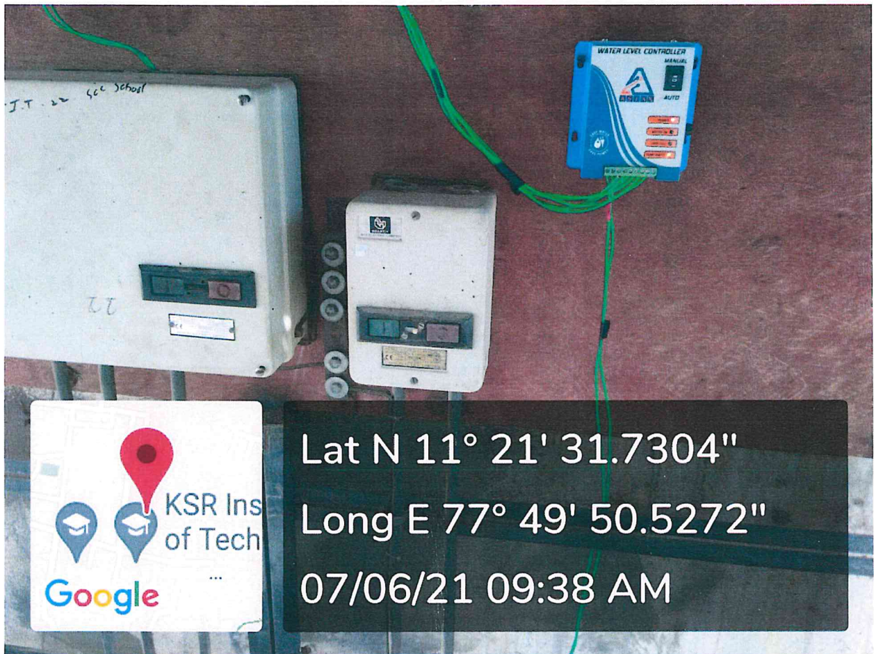
OVERHEAD WATER TANK - WATER LEVEL CONTROLLER
