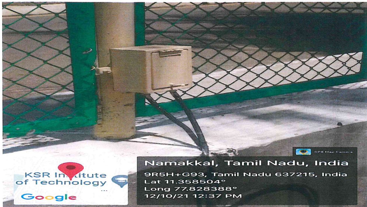
Automatic street light sensor
