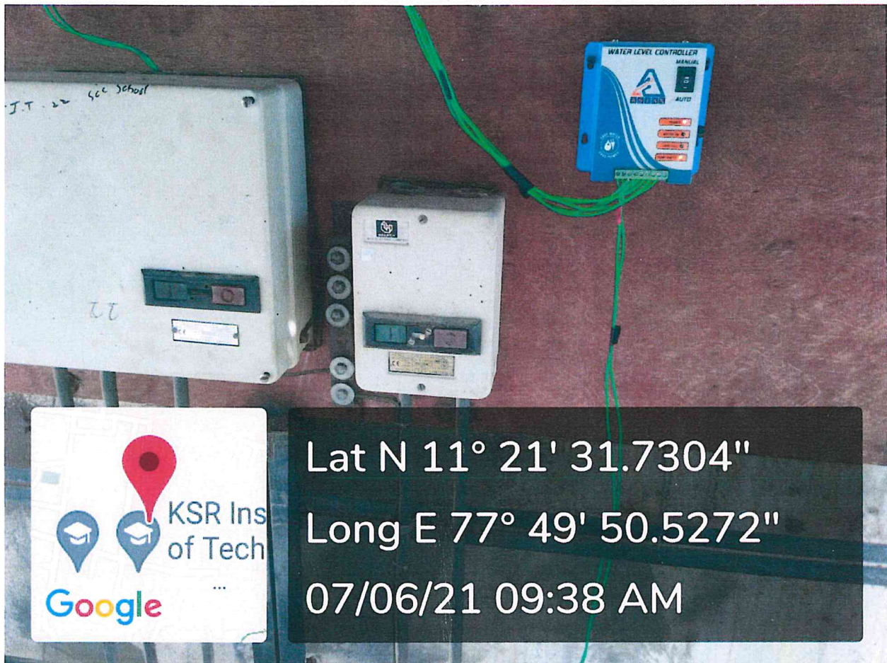
OVERHEAD WATER TANK - WATER LEVEL CONTROLLER
